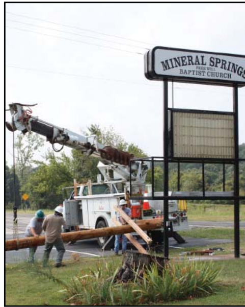
Cookson Hills Electric Cooperative contractors upgrading facilities in the W-W Grocery area north of Muldrow.
