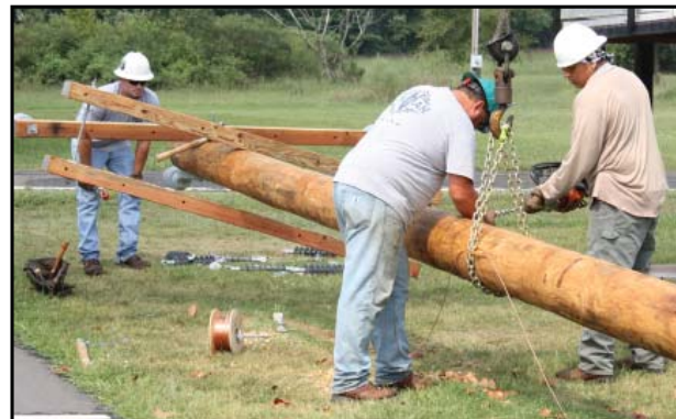
Texoma Powerline Inc. Contractors assembling crossarms on new electric poles near W-W Grocery corner. Photos by: Larry Mattes
